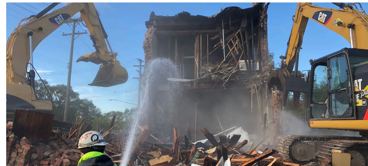
Figure 84: The demolition of Kovacs Bar at the furthest corner of what will be the new bridge plaza site
