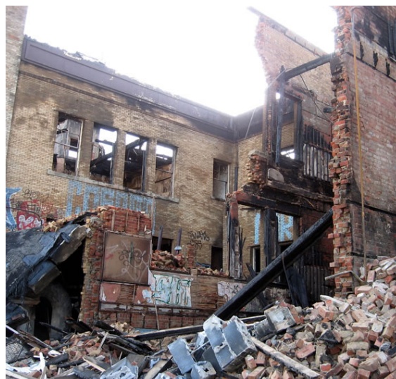
Figure 79: Crumbling interior walls of McMillan School
