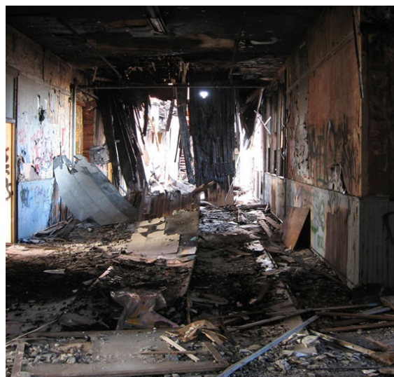
Figure 81: The dilapidated hall way
