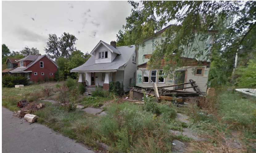
Figure 28 Example of Poor Conditions Houses in the target area located on Ashland Street (Capstone Team)
