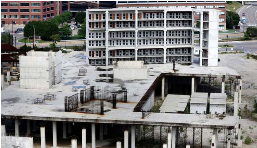
Figure 9: Failed Wayne County jail site on Gratiot (Blanquart)
