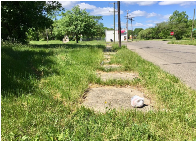
FIGURE 3.1 Condition of sidewalk in Nardin Park
