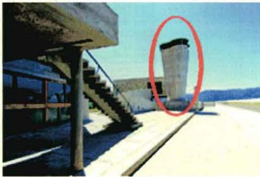
The ventilation stacks are aculptural and not just treated as an afterthought.
