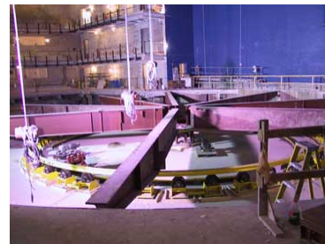
Final layer of the revolving stage's mechanism. The stage itself is installed atop the I-beams.
