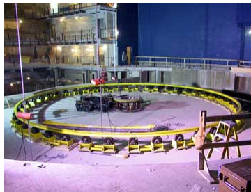
The first layer of the revolving mechanism for the Perelman Theater's turntable stage
